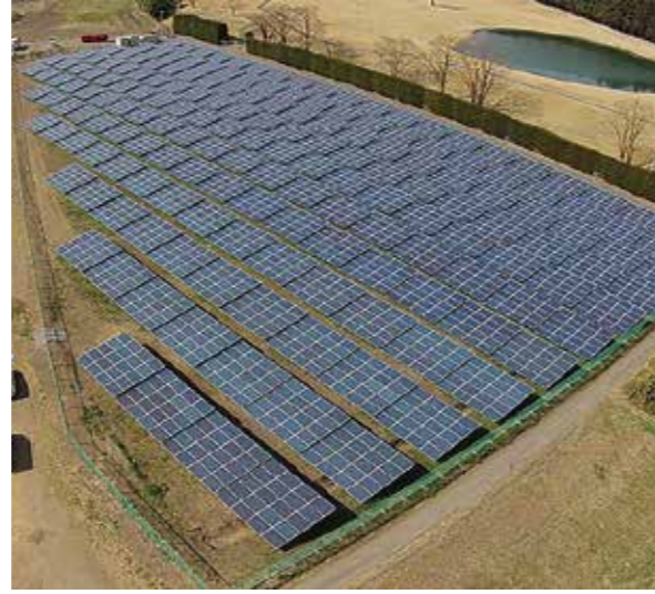
► 875KW PV Station in Takasaki, Japan
