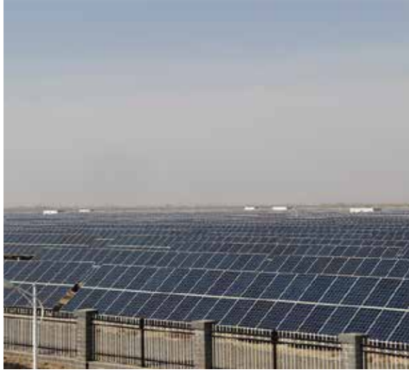
► Optimized 1MW PV Station in Xinjiang, China
