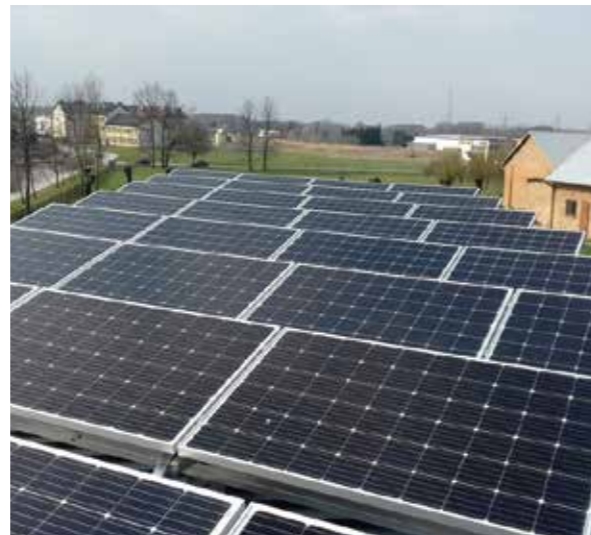
► 10.08KW Rooftop PV Station in Poland
